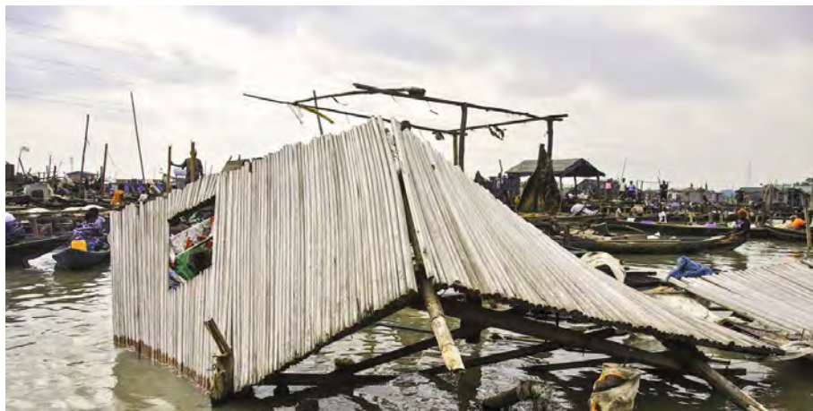
The remains of a waterfront house demolished on the orders of the Lagos State Commissioner for the Waterfront, the Hon. Segun Oniru, during Governor Babatunde Raji Fashola's administration.
